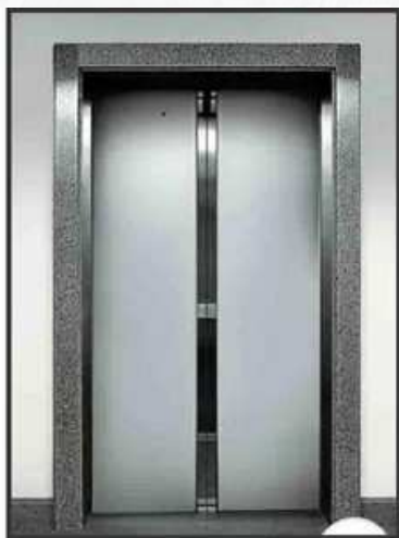
Automatic Center Opening Powder Coated Door
